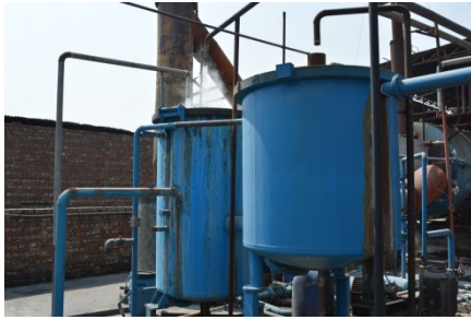
New Condensate Return System
