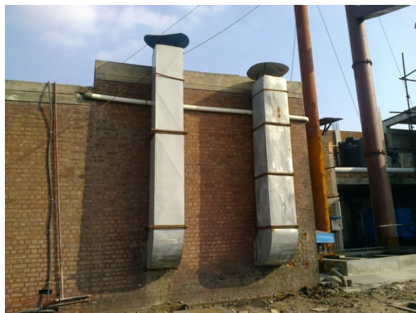
Improved Ventilation in Screen Stripping to reduce inhalation of fumes
