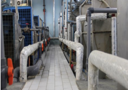
Insulated steam pipes
