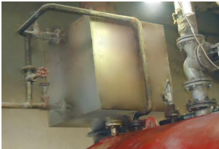
Boiler Exhaust Waste Heat utilized in Wood Furnace
