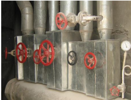
Insulated steam valves
