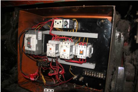
Star-delta drive installed on Ring Frame
